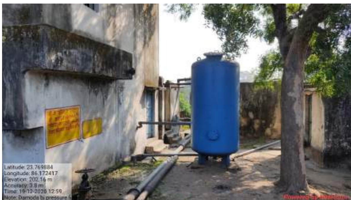
FILTER PLANT IN THE MINE AREA
